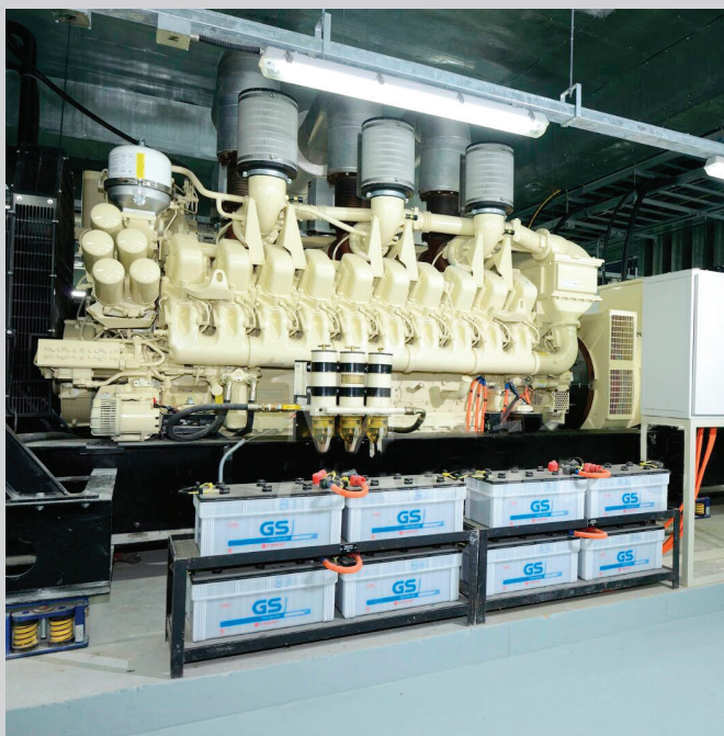
Total 7 set of 11000V Generators inside Genset Room
