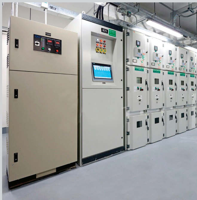
High Voltage Switchboard with Synchronization System
