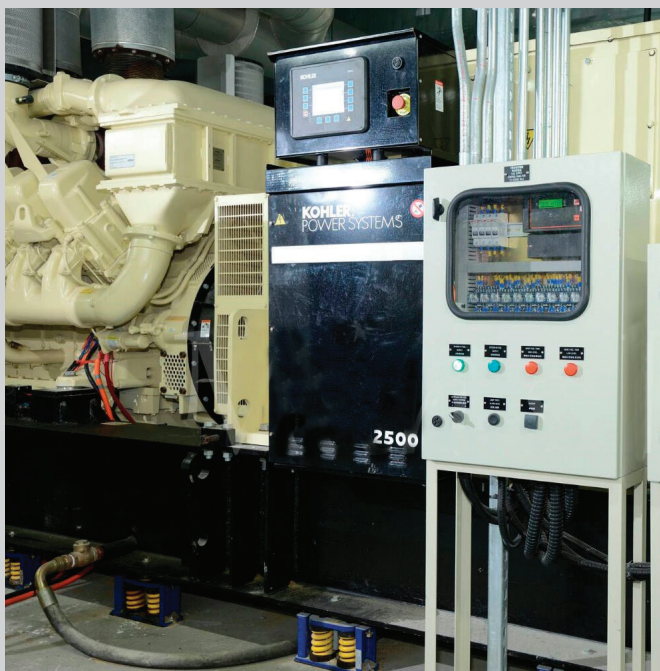
Generator Fuel System Control Panel with Ultrasonic Level Sensor
