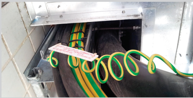
Cable Installed on External Wall
