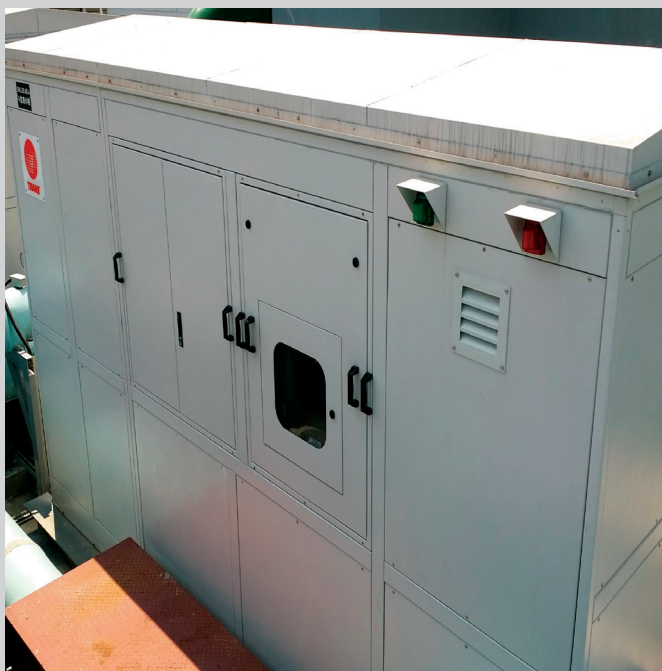
Weather-proofing Enclosure for Chillers
