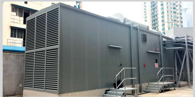
Weather-proof Enclosure for Generators (JEC)
