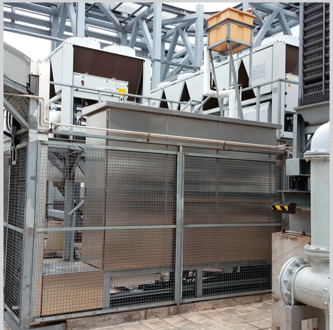
LVSB Installation inside S.S. Enclosure
