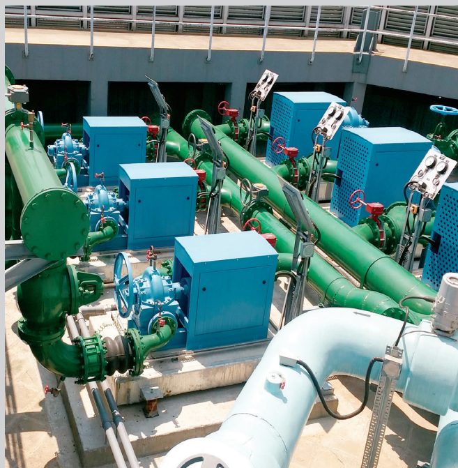
New Condensing Water Pumps System
