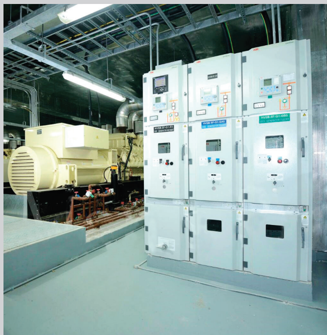
21sets of High Voltage Switchboard for HV Generators
