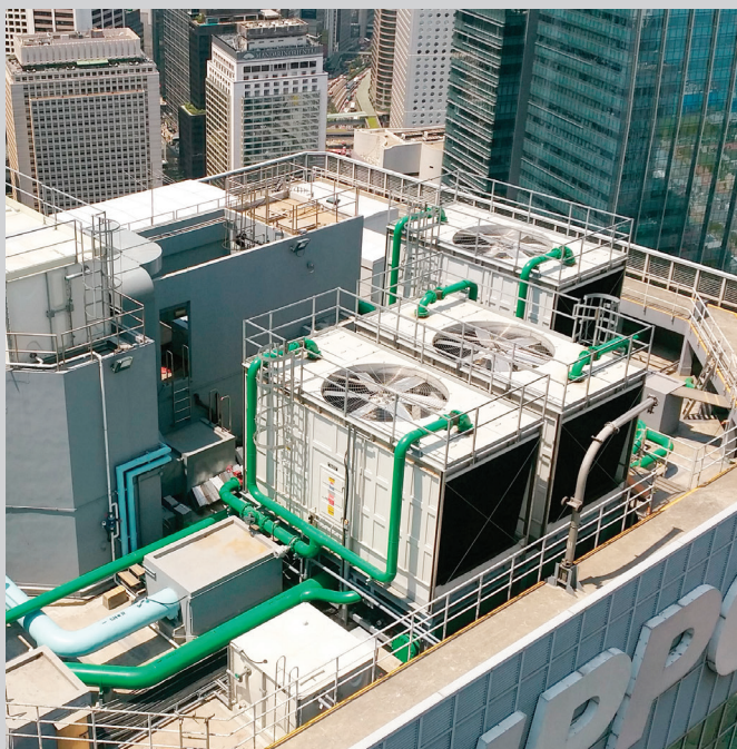
New Installed Chillers with Enclosure and Cooling Tower
